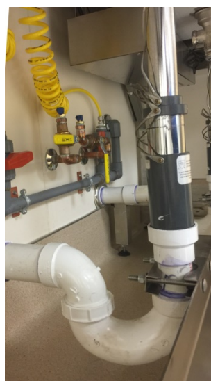
Drain mounted to sink frame cross member
